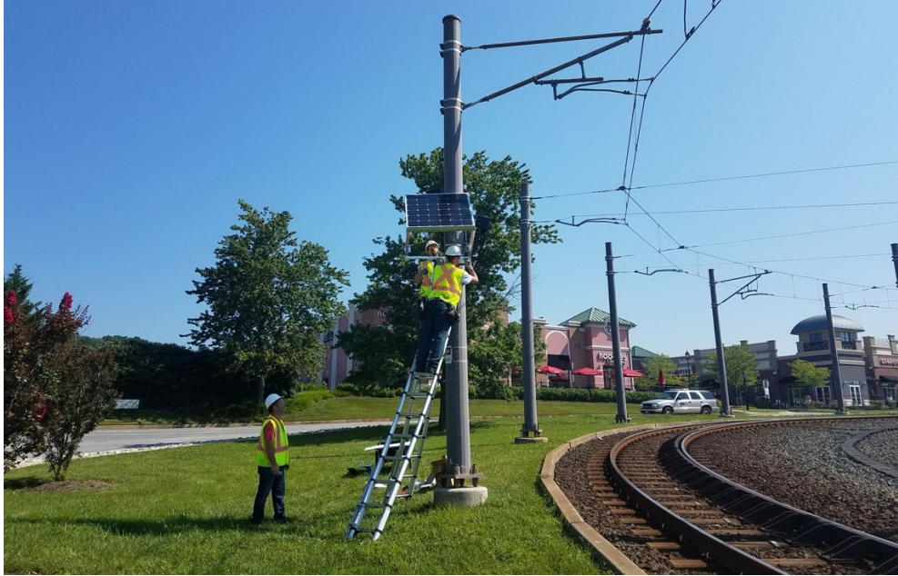
Figure 1: Installation of fixed ZoneGuard™ eRWP system on MTA Baltimore Light Rail Line.
